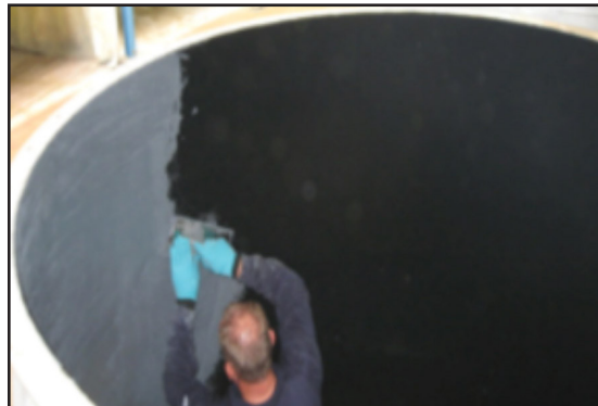
After cleaning, ARC 855 primer was applied by roller and ARC BX1 and ARC BX2 were trowel applied
