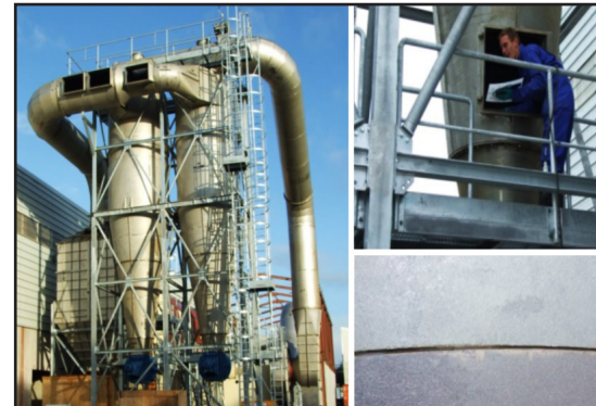
After assembly on site, repeat priming and coating on ID of flanges and weld seams
