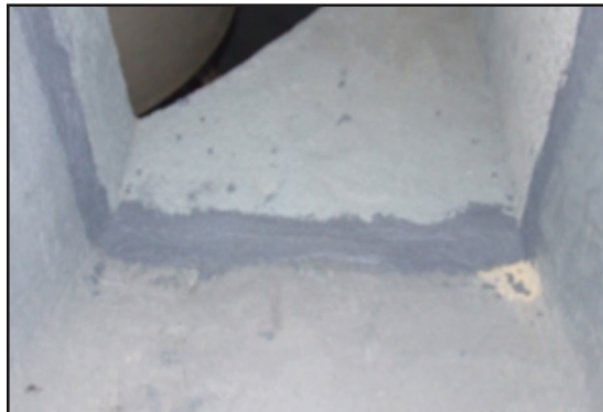
Nearly 100% of coating performed in work shop in 2.5 weeks by 3 applicators working 8-hour shifts
